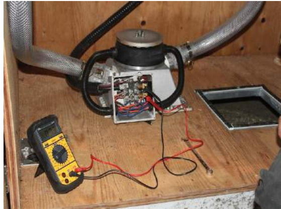
Figure 6 - Turbine installed in turbine house. Water enters through the two clear pipes and drains out under the turbine.
